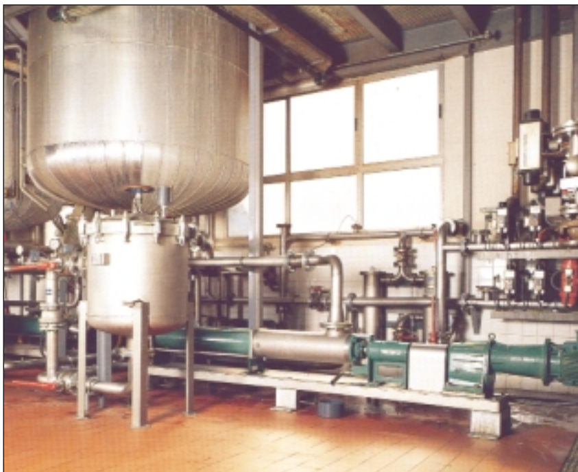
Two NEMO NM Pumps automatically suction lift detergents from two reaction vessels to large reservoir tanks 330 feet away.
